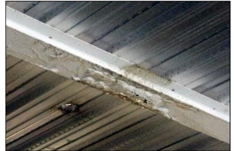
Water damaged intumescent paint
