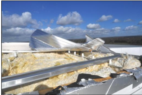
Weather damaged sheet roofing
